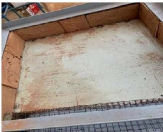
Figure 1. Refractory bricks in the furnace
