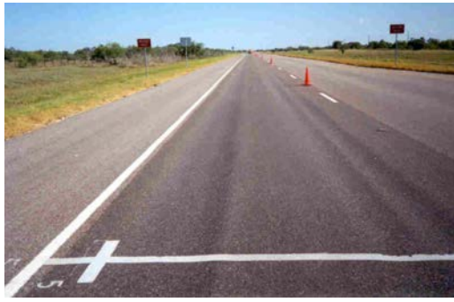
Figure 1. Rutting for a pavement structure [1]
