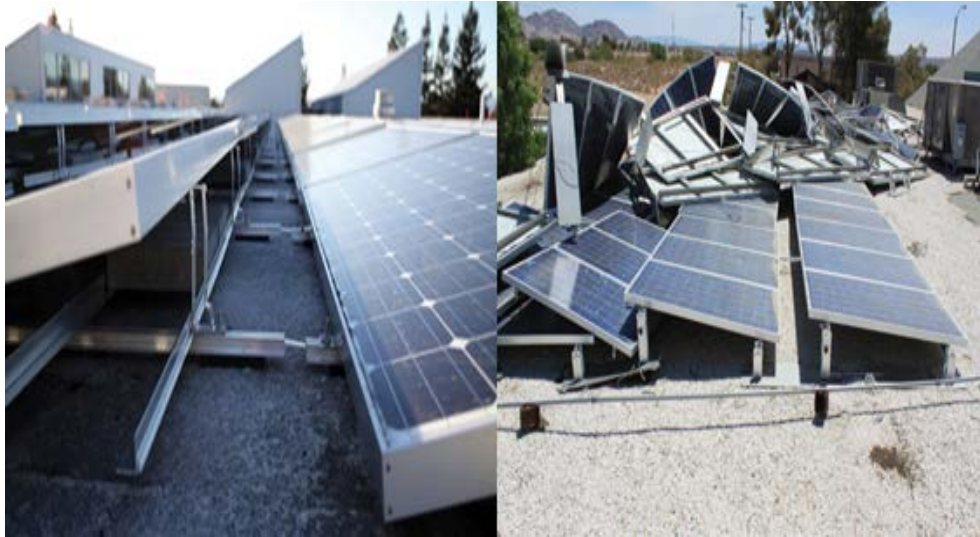
Figure 2. Failure and damage of the mount ground solar tracker caused by strong wind [7]
